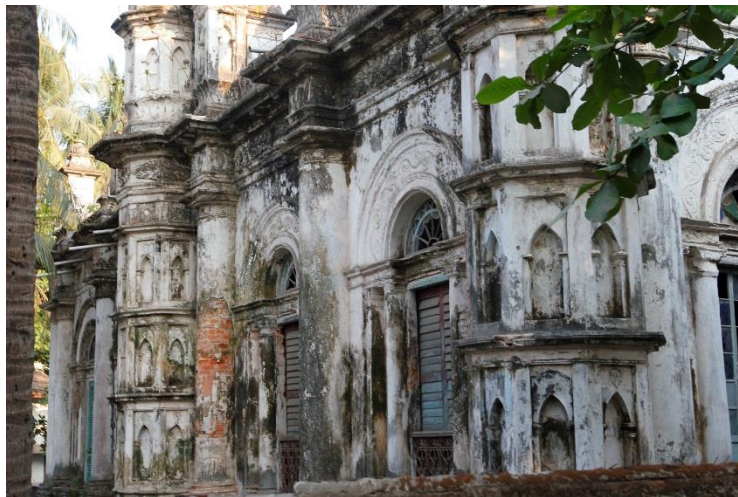
↑ Sittwe's once imposing main mosque has fallen into a state of disrepair and decay. Shuttered since 2012, police guards and barbed wire fences prevent anyone from entering, March 2016. ©Amnesty International.
